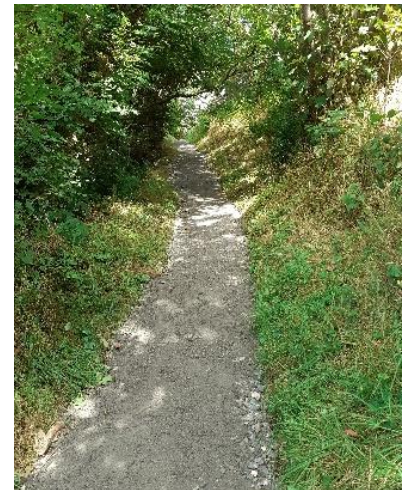
Right: The footpath below the cycle barrier at Bryn y Mor after resurfacing. (Photo Len Kersley)
